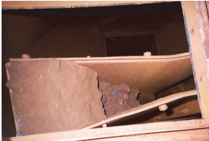
Figure 12. Partially blocked cutter aperture in a Vezin divider.
