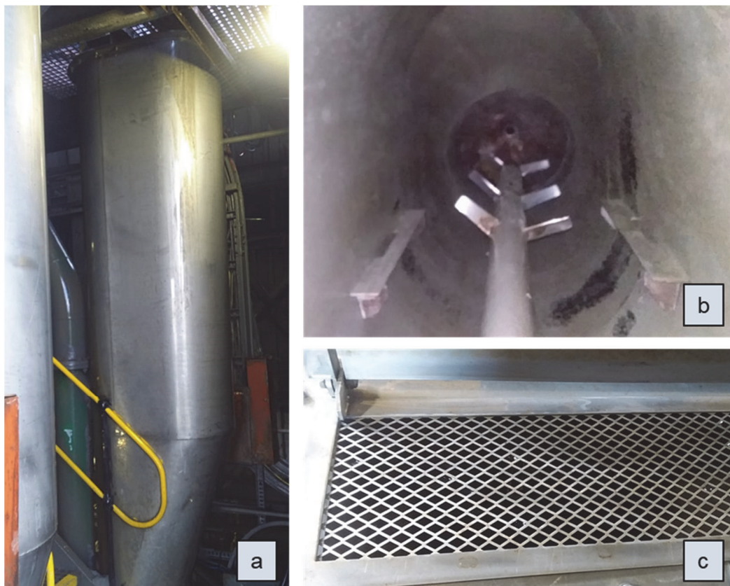
Figure 2. Day Tank – a. Oval Tank Design; b. Off Centre Agitator inside Day Tank; c. Sampler Inspection/Safety Grid.
