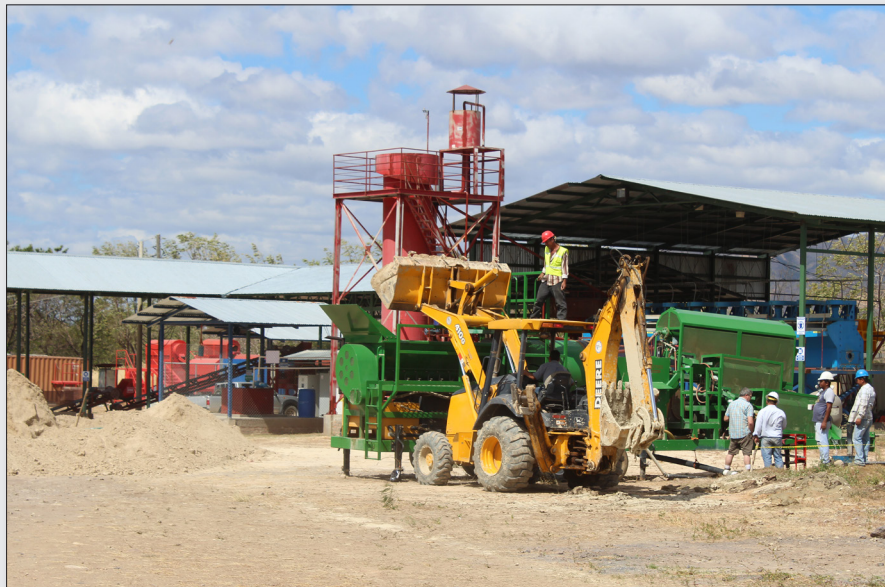
Figure 7. Mercury Recovery Plant (MRP) being loaded by tailings (Nicaragua).
