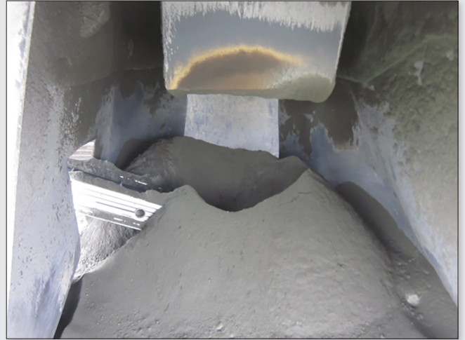
Figure 12. A drill cuttings cone as viewed from under the dust curtain, with the RAS conveyor belt in place.
