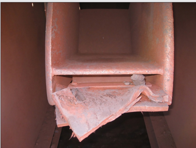
Figure 15. Poor condition of the rubber skirt on the bottom of a cross-belt cutter.
