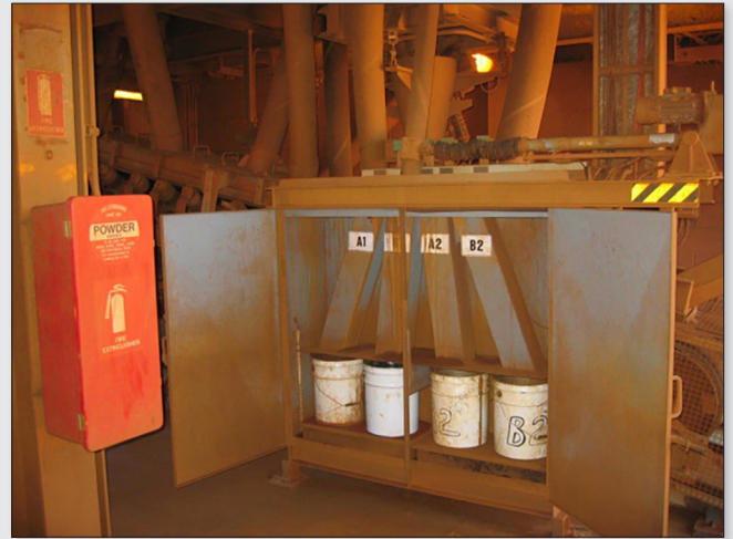
Figure 17. Duplicate sampling system installed in a sample station.
