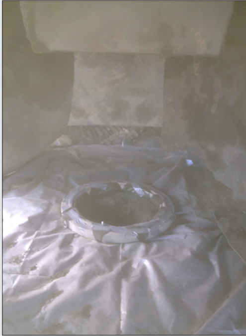
Figure 10. Tarp laid on the ground around the concrete ring, which surrounds the blast hole.
