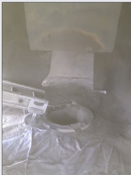
Figure 11. Primary sampling conveyor is pushed through the opening in the dust curtain and placed next to the mouth of the blast hole.
