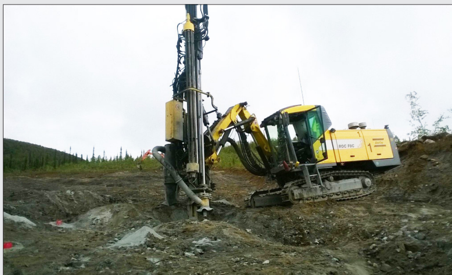
Blast hole drilling in Svappavaara, one of the more interesting sampling situations we face at LKAB today.
