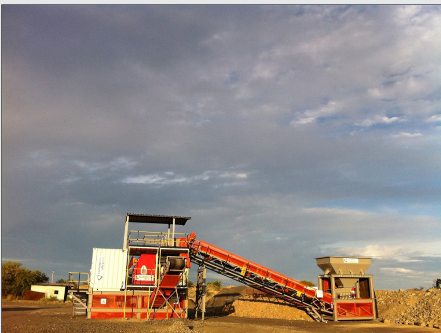
Figure 3. On-site containerised, semi-mobile chute-type sorter installation.
